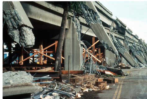
A highway on two levels, that collapsed in the Northern California earthquake of 1989
